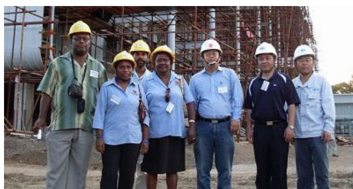
Department of Labour & Industrial Relations officials with Ramu NiCo Management (MCC) Ltd. officers on site tour after Safety brief session
